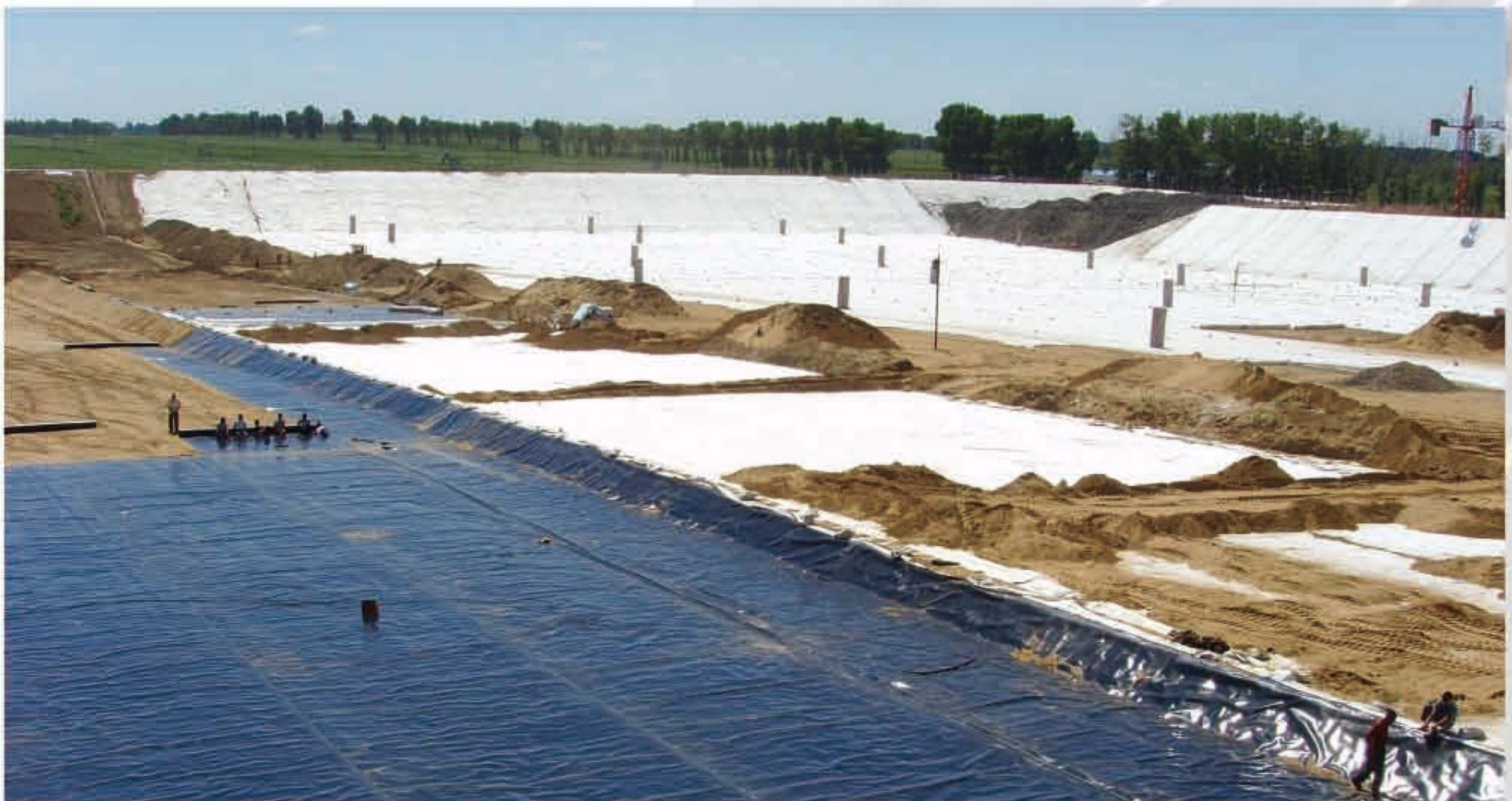
松原垃圾填埋场土工膜铺设现场 Geomembrane installation site of Songyuan Landfill
