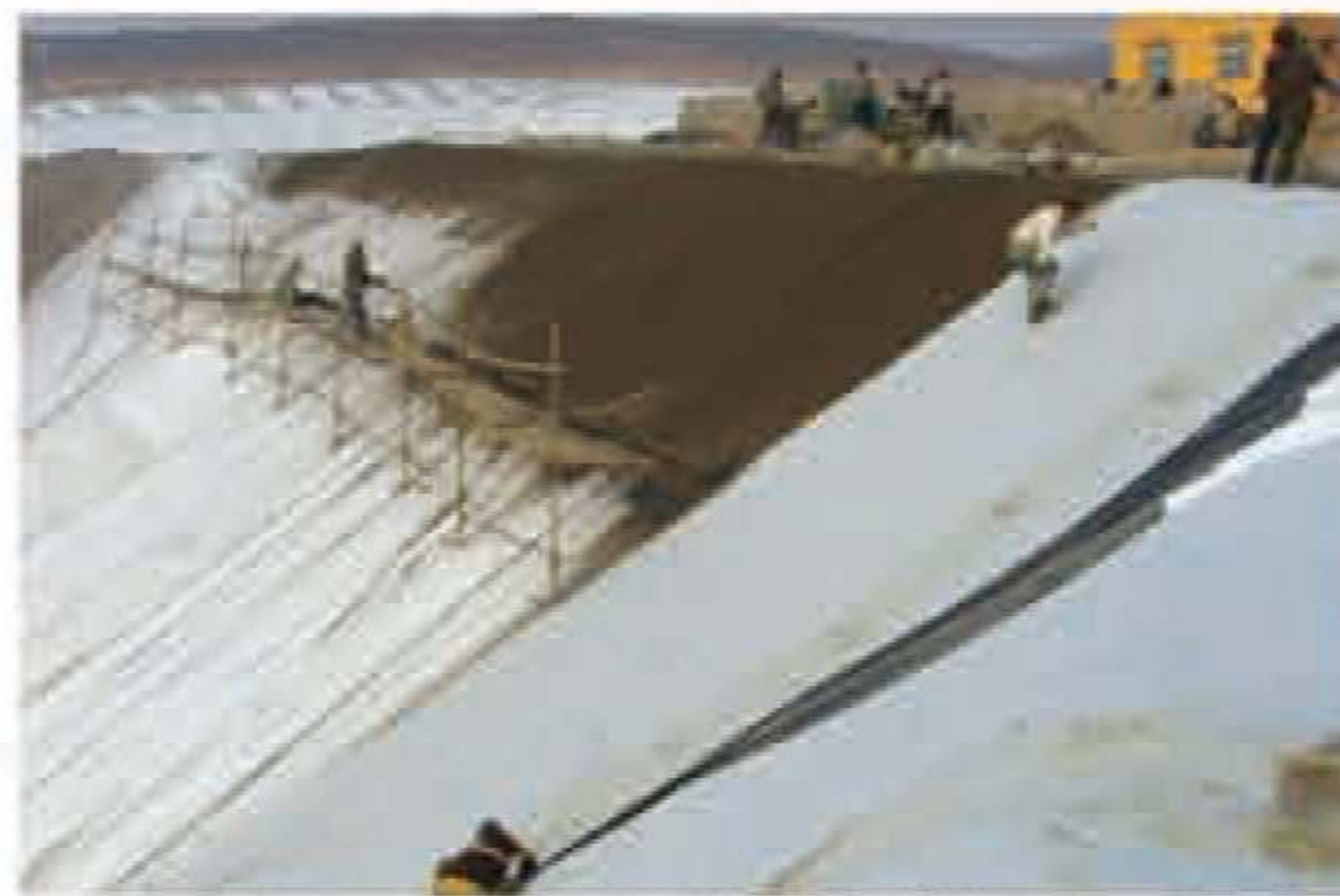
HDPE土工膜在贵州垃圾填埋场中的应用 HDPE geomembrane in Guizhou garbage burial site
